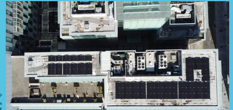
Solar PV panels Central Quay
